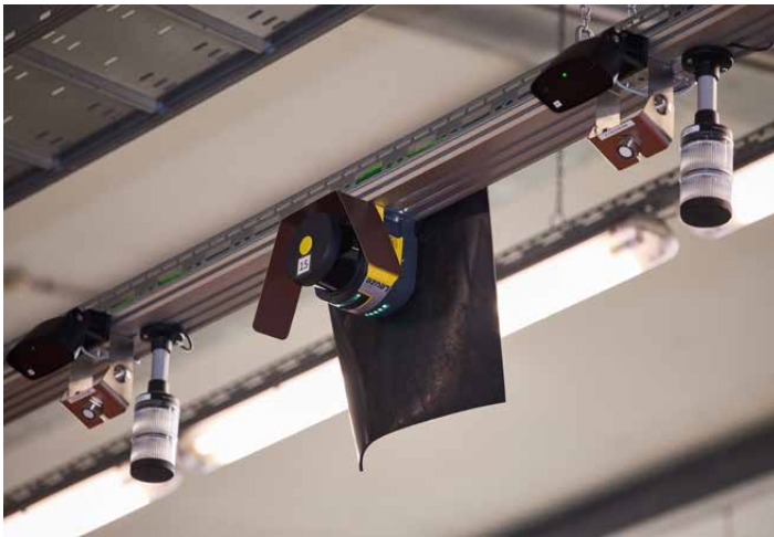
A view of the safety technology in the transfer area: An RSL 400 safety laser scanner from Leuze (center) generates a protective field that covers two transfer stations at the same time. In addition, an ultrasonic sensor and a radar sensor are mounted on each station (to the left/right of the scanner). An illuminated display shows the status for each station.
